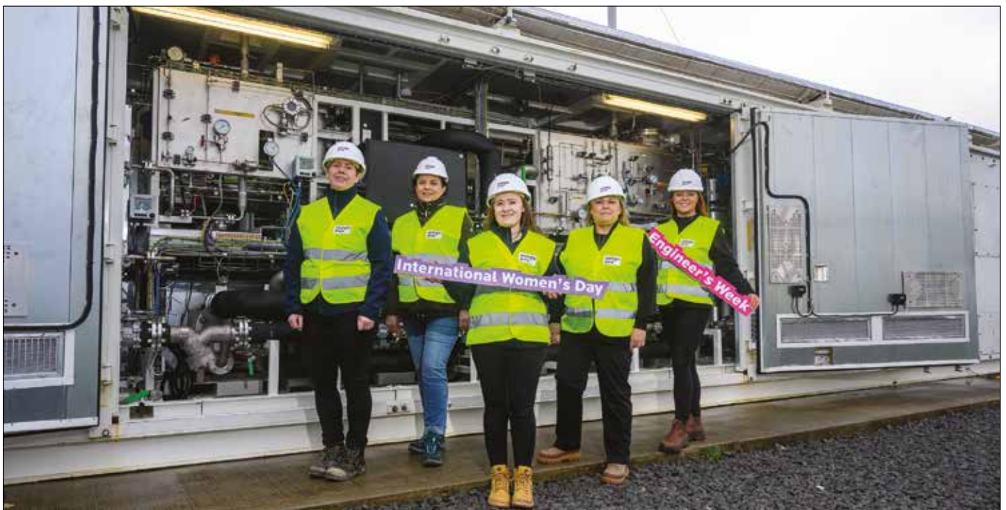
Energia Group shares insights from women working in a variety of roles in the Energy sector this International Women's Day as part of STEP's Engineers Week. Pictured at the Group's Hydrogen Production facility at the Long Mountain Wind Farm, (L-R) Sara Tinsley, Planning and Environmental Consents Manager and Annabel FitzGerald, ESG & Corporate Communications Manager; Susan Glascott, Health, Safety & Environment Manager; Rosy Billingham, Community Engagement and Communications Manager; and Rachael O'Boyle, Operations Engineer in the Renewables Operations Department.
