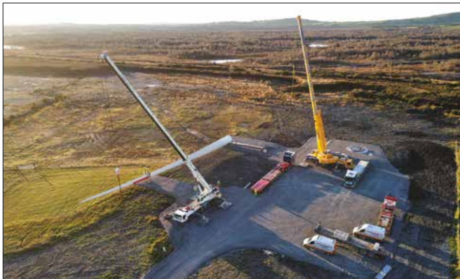
Turbine parts, including towers, nacelles, hubs and blades, are being delivered under Garda escort from Galway Port to the Yellow River site.
